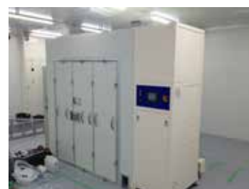
Temperature and humidity control
