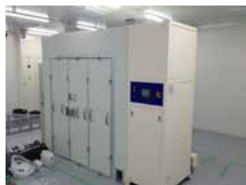
Temperature and humidity control
