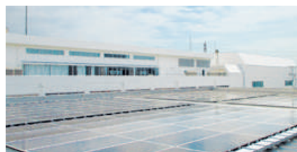
The solar power system on the roof of Building 6 at the head office began operations in July 2024.
