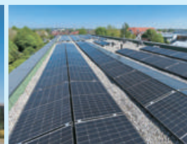
Solar panels on the roof
