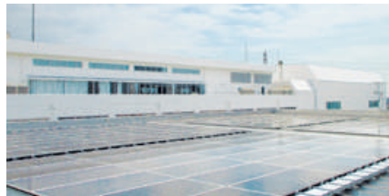
The solar power system on the roof of Building 6 at the head office began operations in July 2024.
